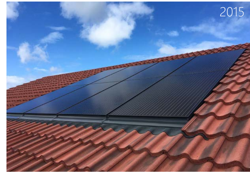
Clearline fusion Roof integrated solar photovoltaic panels
