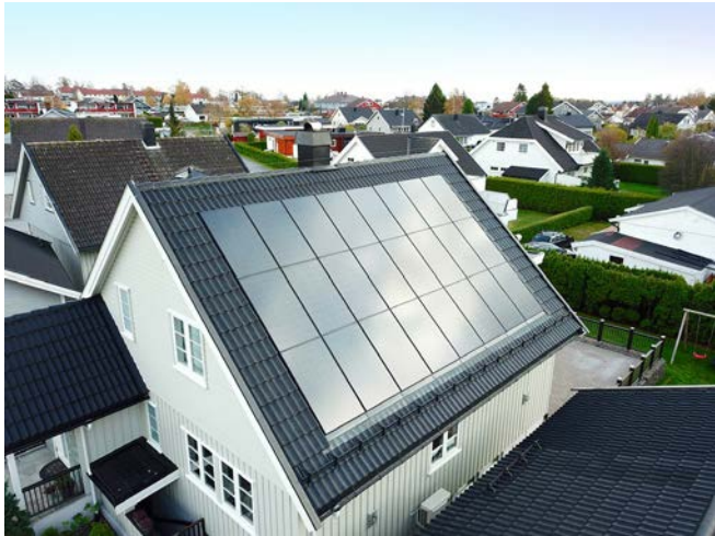
Norway, Tonsberg Retrofit family home installed by Bluetec AS
